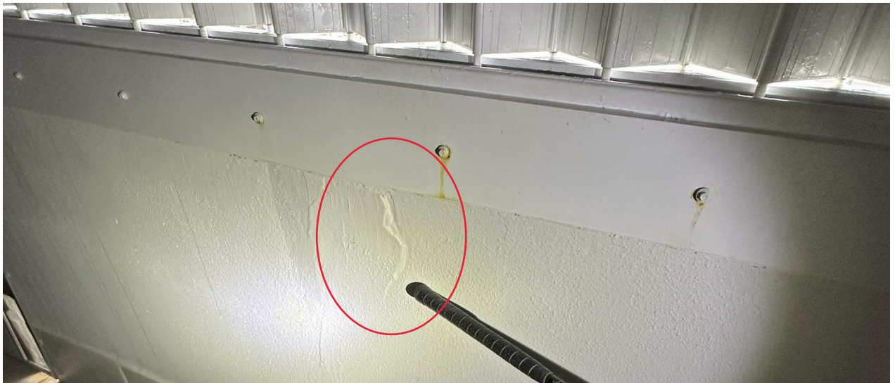
Photo 21: Balcony Parapet Wall, Concrete Spall.
