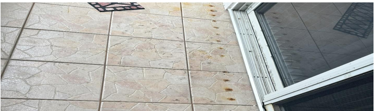
Photo 26: Balcony Floor, Corroding Unremoved Fasteners.
