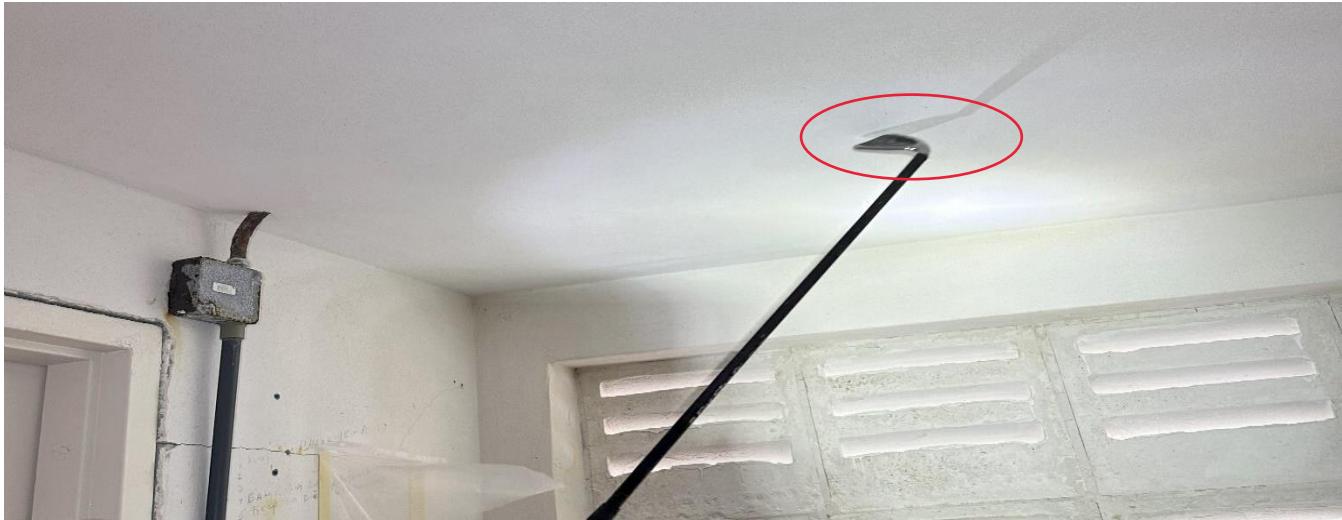
Photo 17: Pool Pump Room Ceiling, Concrete Spall.
