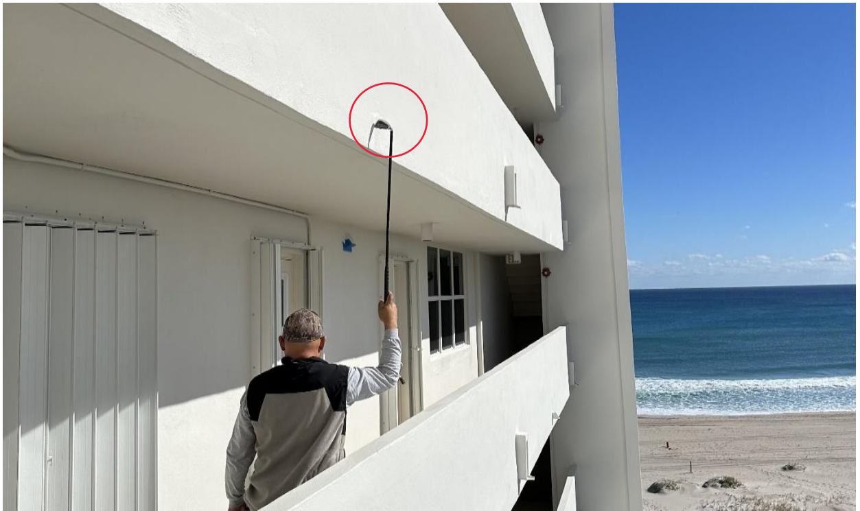
Photo 27: South Elevation Walkways, Parapet Wall Spalls.
