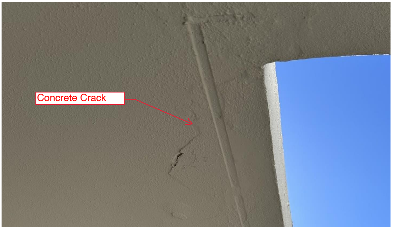
Photo 29: South Elevation Walkways, Ceiling Concrete Crack.
