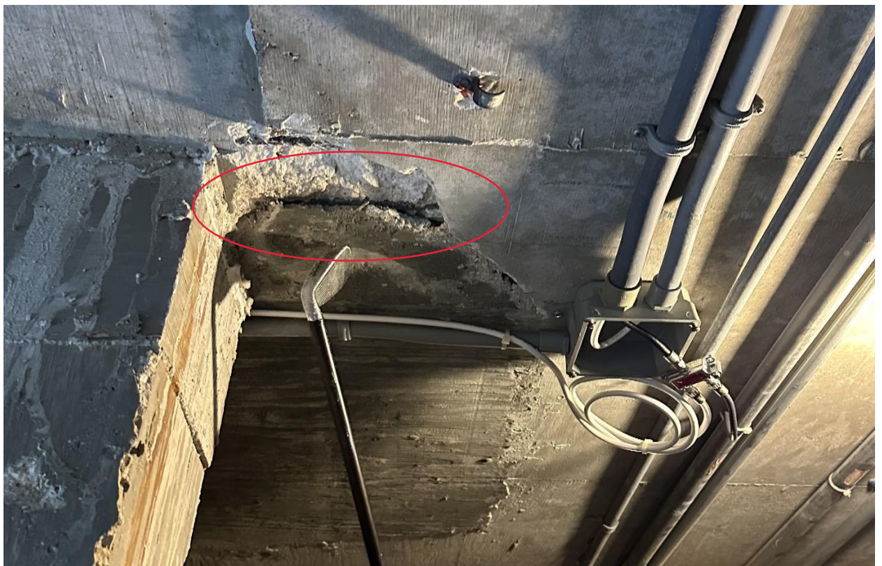
Photo 30: Pump Room, Ceiling Spall with Exposed Rebar.
