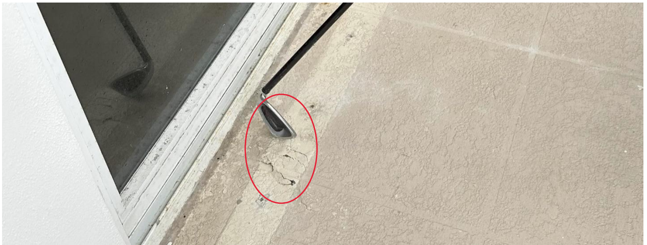
Photo 22: Balcony Floor, Concrete Spall Caused by Unremoved Fasteners.
