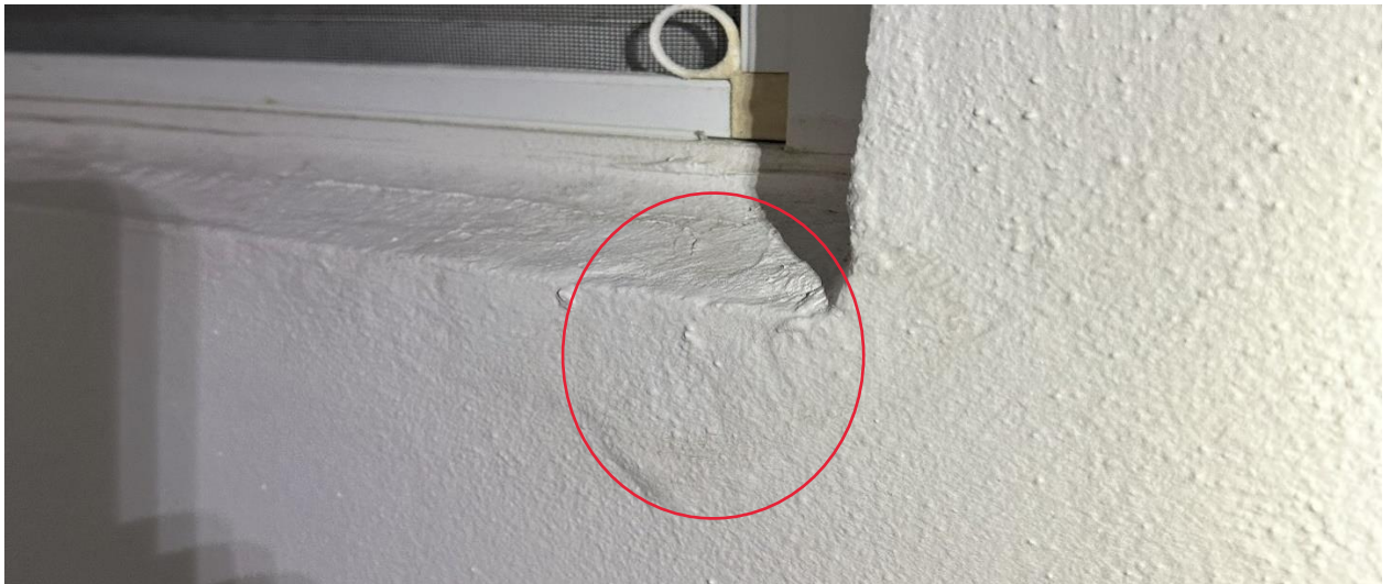
Photo 24: Balcony Window Sill, Concrete Spall.
