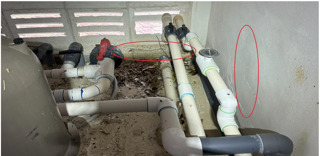
Photo 18: Pool Pump Room Floor, Wall Spalls.
