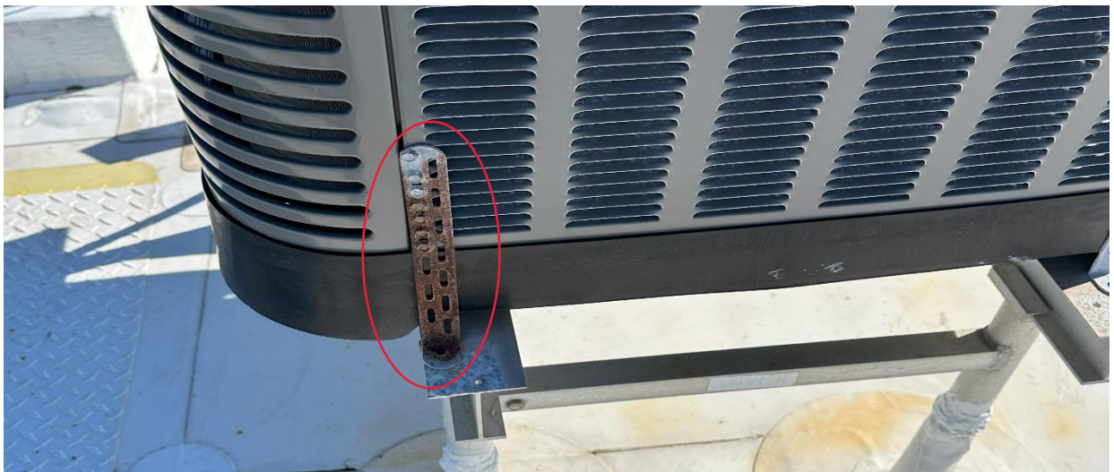
Photo 10: AC Strap Corrosion Damage.
