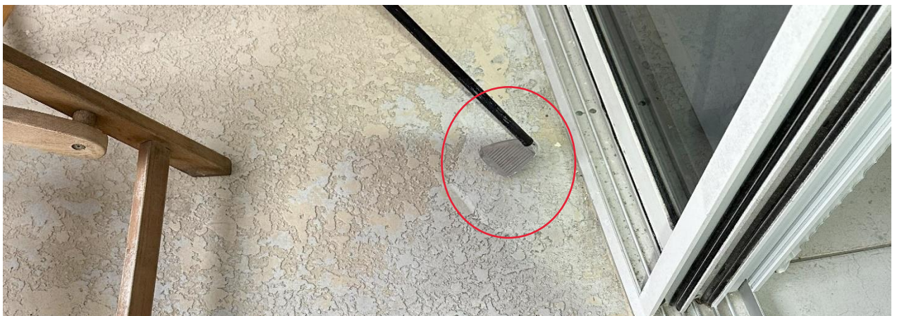
Photo 23: Balcony Floor, Concrete Spall.
