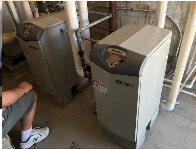
Hot Water Heaters & Boilers
